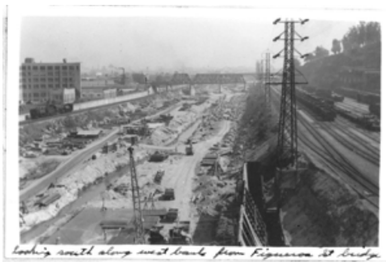
Figure ES-2 The LACDA Project Under Construction, Downstream of Arroyo Seco Confluence 1940
